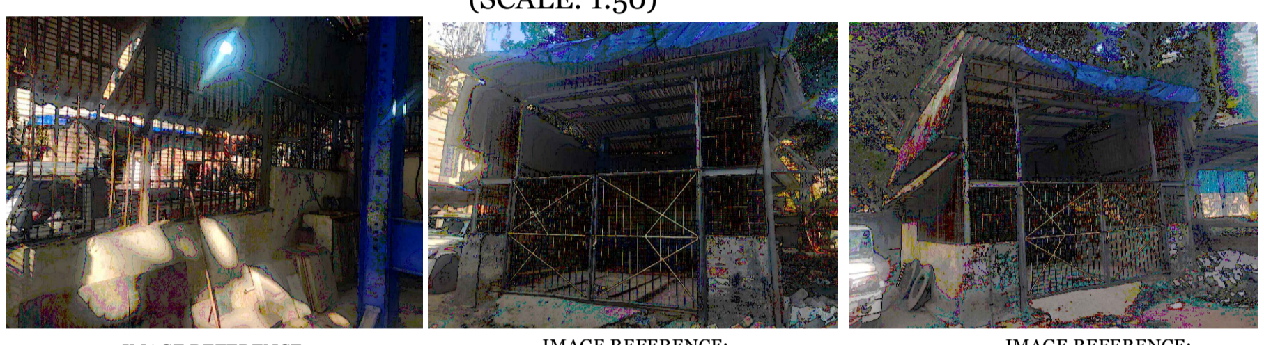
IMAGE REFERENCE: WALL HEIGHT DIFFERENCE OF WESTERN ELEVATION IMAGE REFERENCE: GATE OF SHED IMAGE REFERENCE: EXISTING SHED
